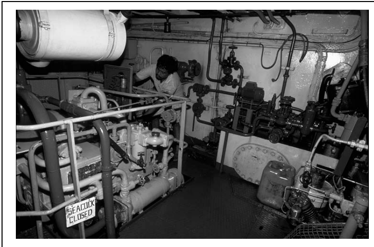
Engine room of ATSA I.
