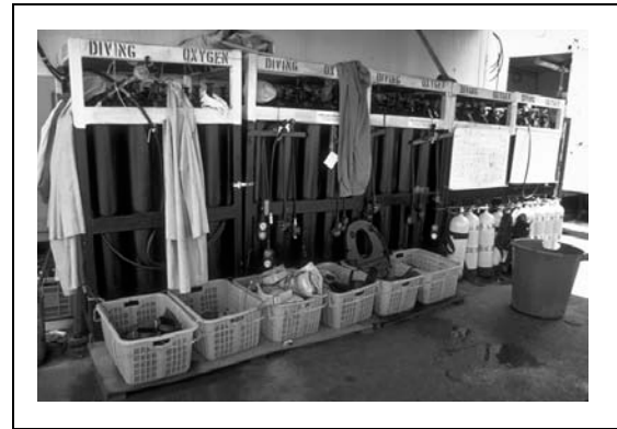
Oxygen racks for surface decompression.
