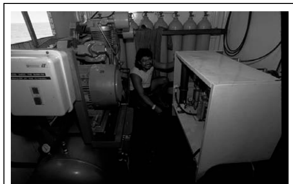
The compression room.
